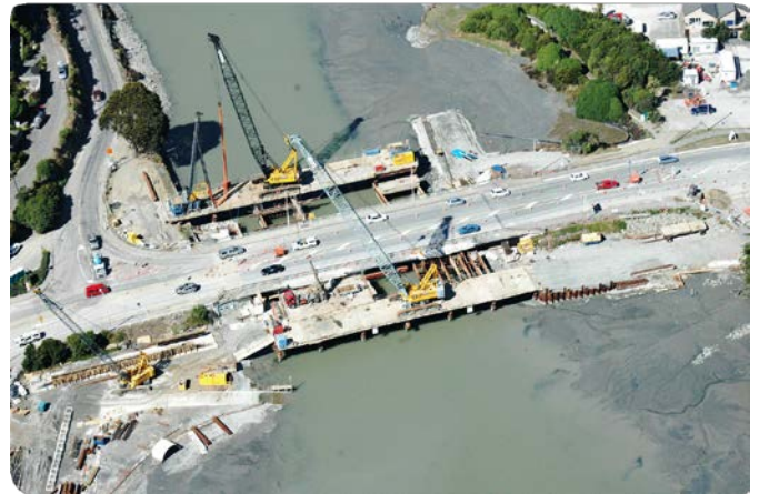
Above: Ferrymead Bridge, Christchurch, under redevelopment. This photo, taken soon after the February 2011 earthquake, shows extensive riverbank damage and liquefaction in the area. Photo credit: H.A. Cowan.
