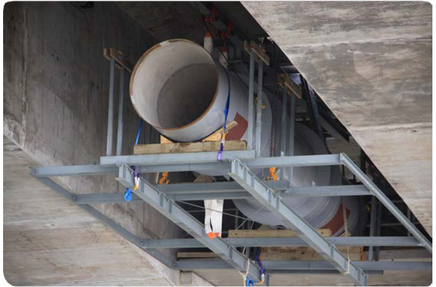
Above: New watermain under construction beneath Mangere Bridge, Auckland. Collaboration is often required between different infrastructure owners when new construction or maintenance is planned. Credit: Watercare Services Ltd
