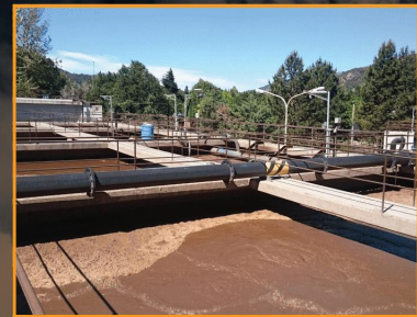
Biological reactors at the municipal wastewater treatment plant at San Martin de los Andes, Argentina, continued to function without problems despite receiving 2 cm of ashfall from the 2015 eruption of Calbuco volcano, 165 km away in Chile. This was partially because the town's storm drains and sewers are well separated, so very little ash entered the plant in raw wastewater. Photo credit: Daniel Blake
