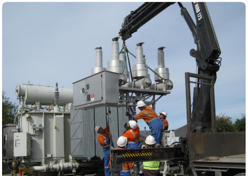
ABOVE: INSTALLATION OF A TEMPORARY TRANSFORMER AT THE NEW BRIGHTON SUBSTATION, CHRISTCHURCH, FOLLOWING THE FEBRUARY 2011 EARTHQUAKE. AN EMERGENCY 66kV OVERHEAD LINE WAS ALSO QUICKLY BUILT TO SUPPLY THE AREA. CREDIT: ORION NEW ZEALAND LIMITED
