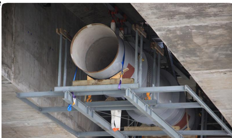
ABOVE: NEW WATERMAIN UNDER CONSTRUCTION BENEATH MANGERE BRIDGE, AUCKLAND. COLLABORATION IS OFTEN REQUIRED BETWEEN DIFFERENT INFRASTRUCTURE OWNERS WHEN NEW CONSTRUCTION OR MAINTENANCE IS PLANNED. CREDIT: WATERCARE SERVICES LTD
