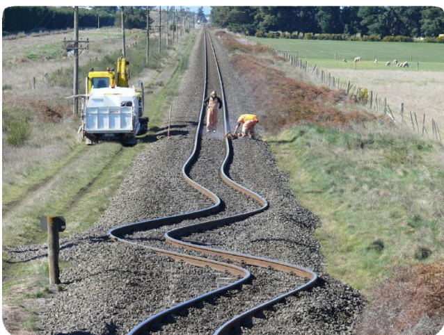
ABOVE: LINES DAMAGED IN CHRISTCHURCH EARTHQUAKE. KIWIRAIL CARRIED OUT QUICK REPAIRS AT THIS AND OTHER DAMAGED SITES
