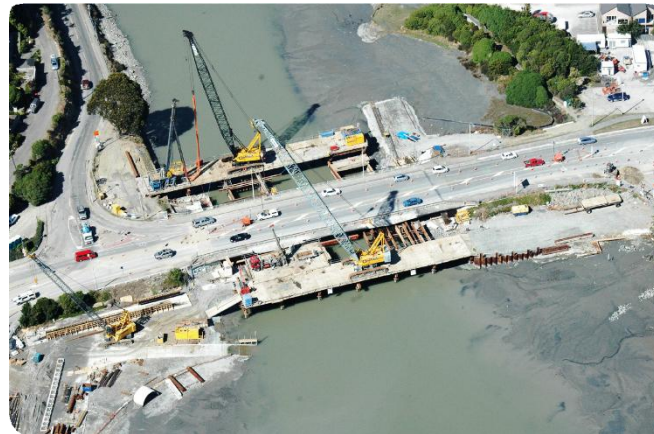
ABOVE: FERRYMEAD BRIDGE, CHRISTCHURCH, UNDER REDEVELOPMENT. THIS PHOTO, TAKEN SOON AFTER THE FEBRUARY 2011 EARTHQUAKE, SHOWS EXTENSIVE RIVERBANK DAMAGE AND LIQUEFACTION IN THE AREA. CREDIT: H.A. CURRAN
